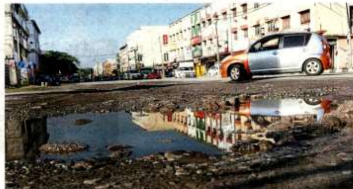
There are many potholes along Jalan Tengku Badar in Port Klang. — KK SHAM/The Star
